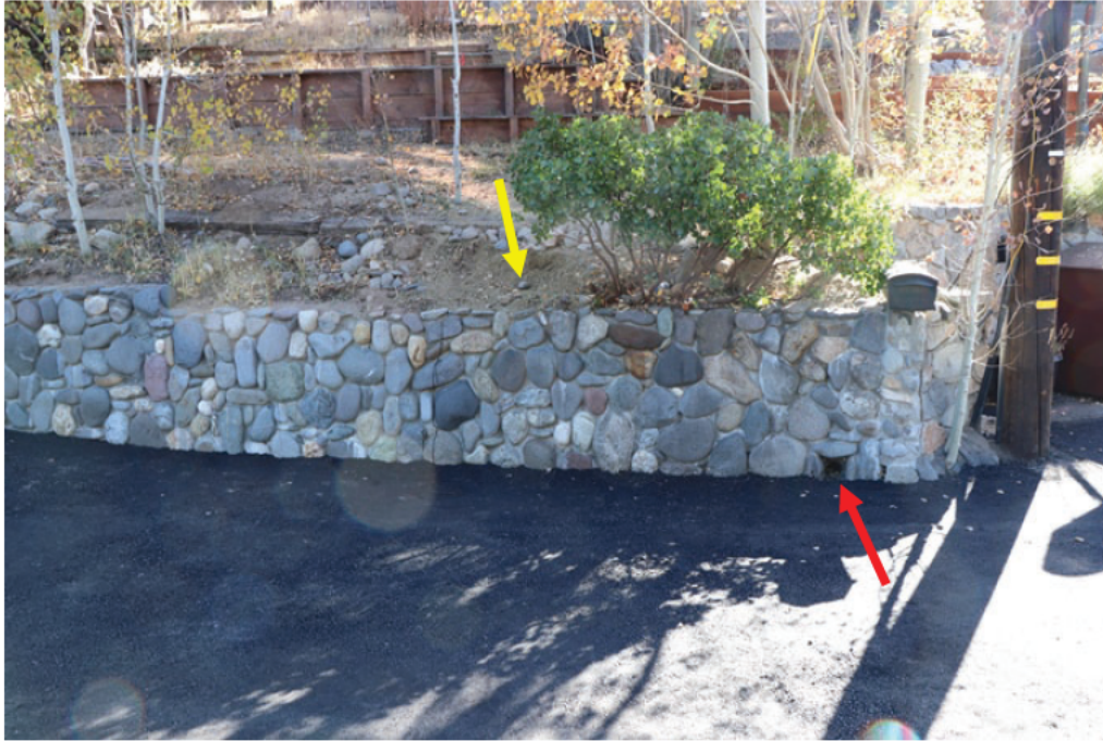
Photo 5: View of the retaining wall outlet drain (red arrow) in relation to the excavation behind the wall (yellow arrow).
