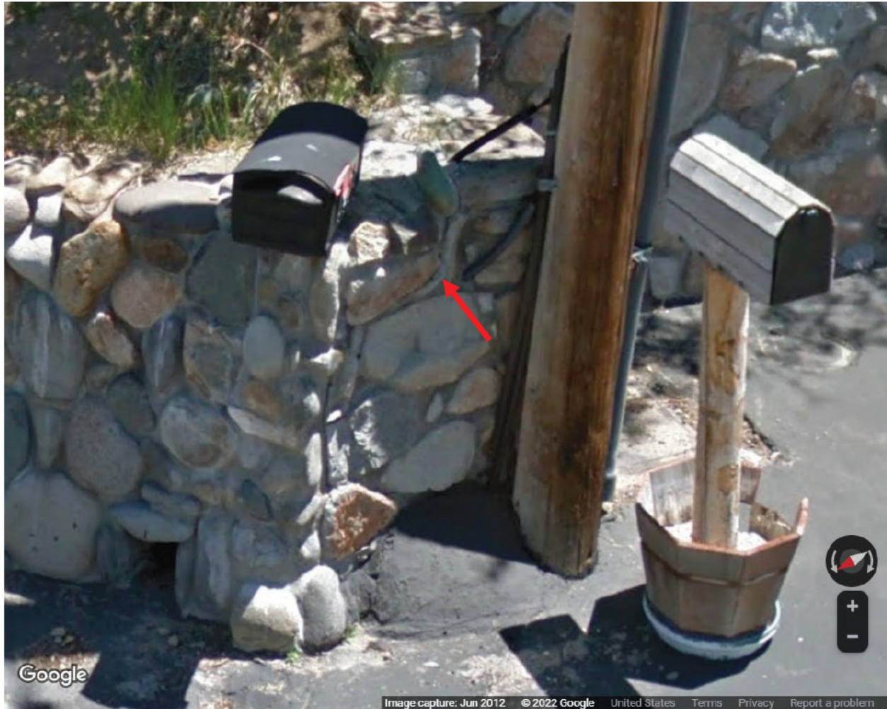
Photo 13: Google Street View Image dated June 2012. Note wall crack is evident in image.
