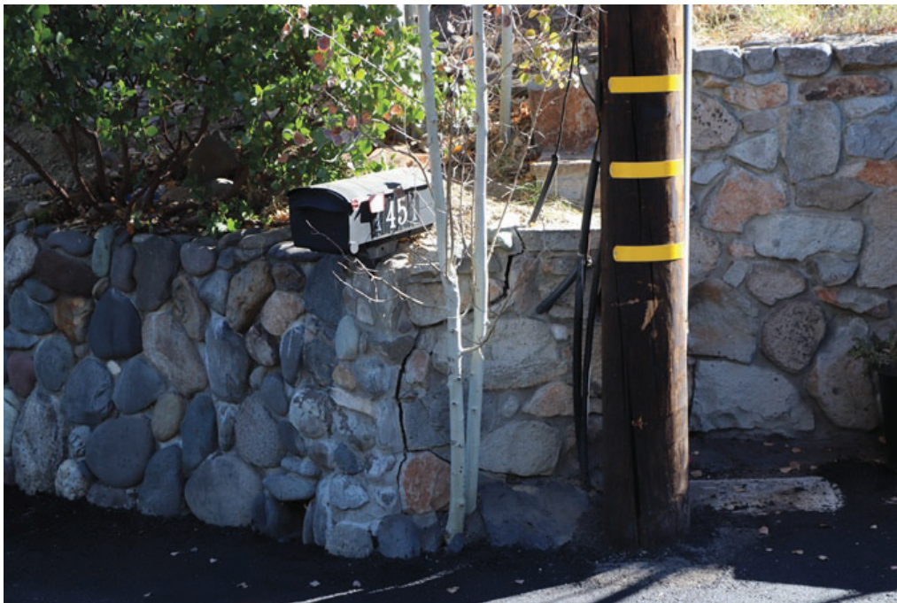
Photo 8: Crack in the neighbor's retaining wall, near where it joins the claimant's wall.
