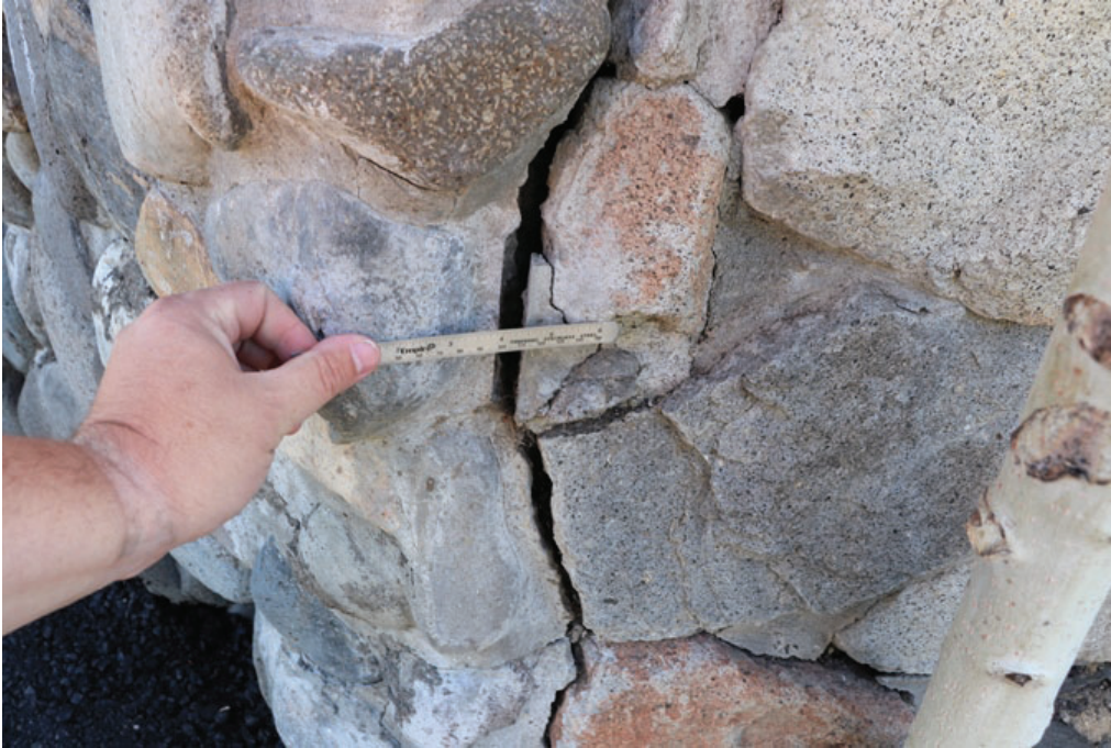
Photo 11: Closer view of the crack in the neighbor's retaining wall.
