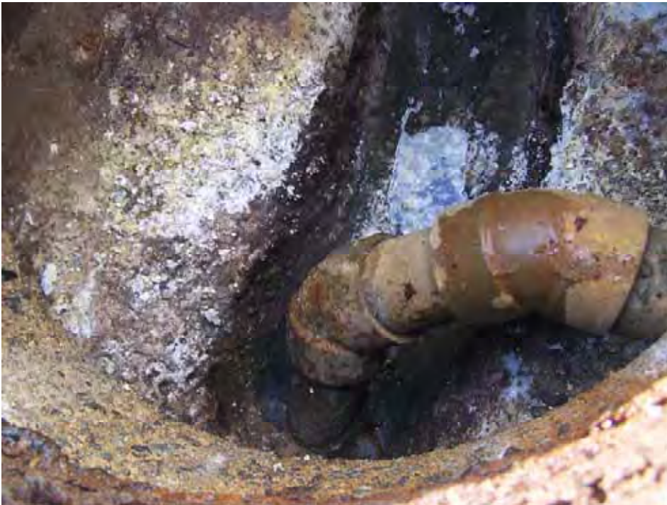
Description: Crumbly Concrete Bench (3/4" Penetration)
