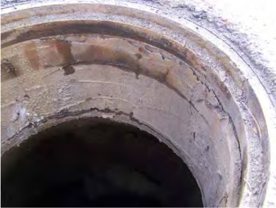
Description: Mortar Coating Pulling Away From Chimney
