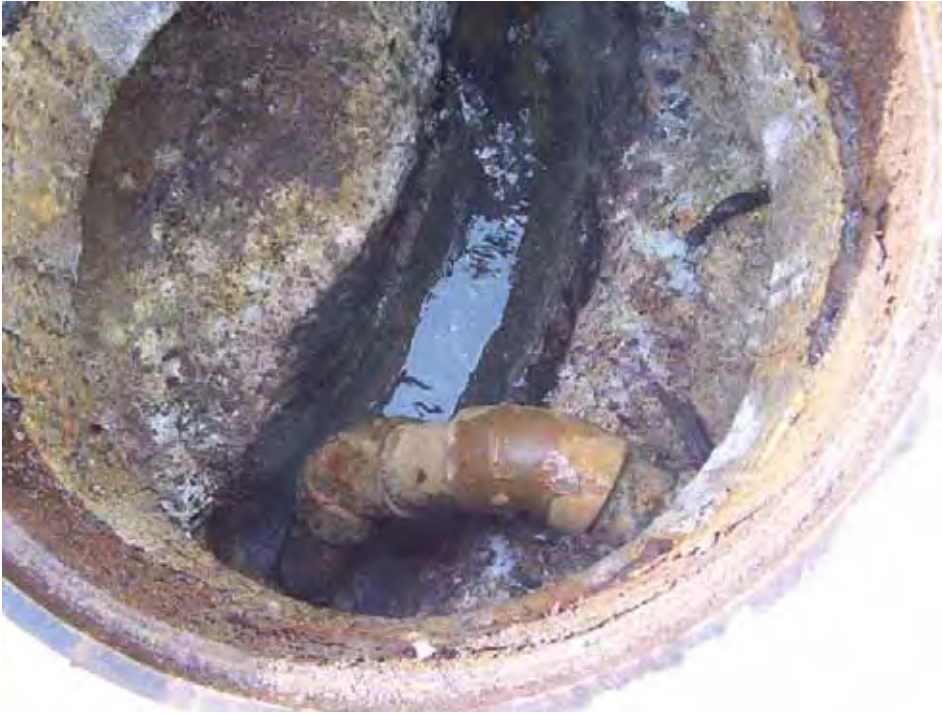
Description: White and Yellow Deposits on Unlined Concrete
