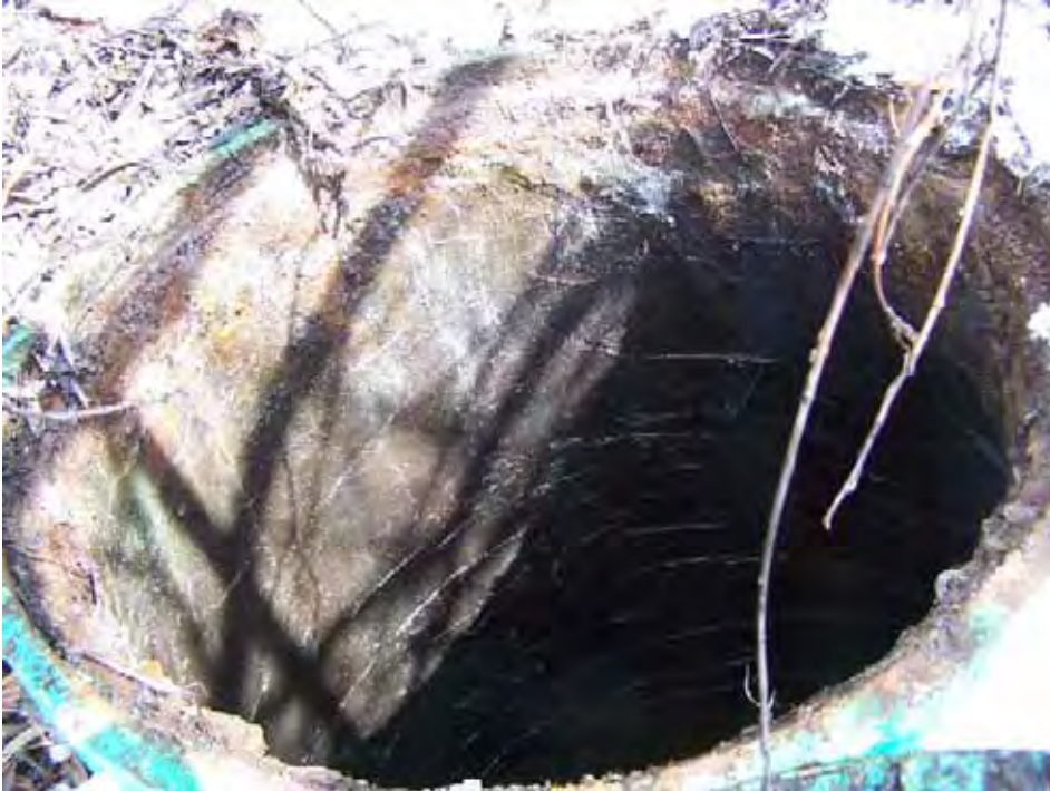
Description: Light Roots Intrusion, Unlined Concrete
