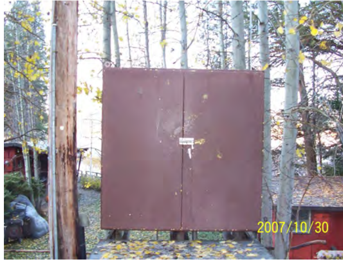
Figure 4-1. Electrical Cabinet at Beecher Pump Station
