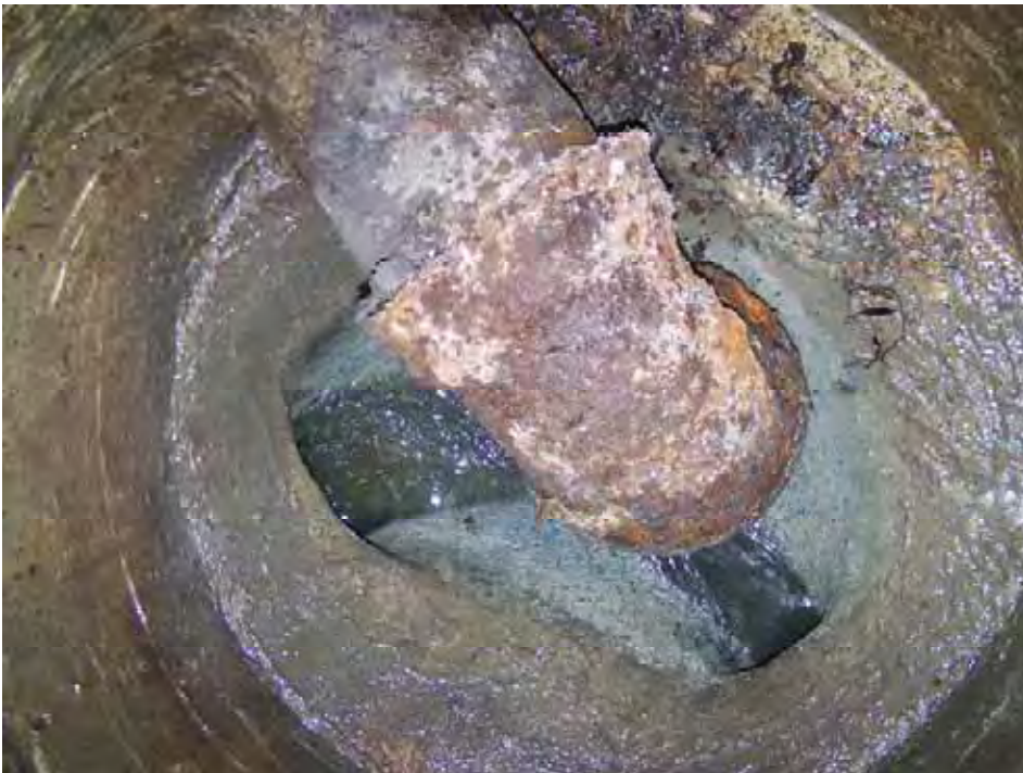
Description: 90 Deg Bend on End of Forcemain, a Lot of Turbulence during Pump Discharge
