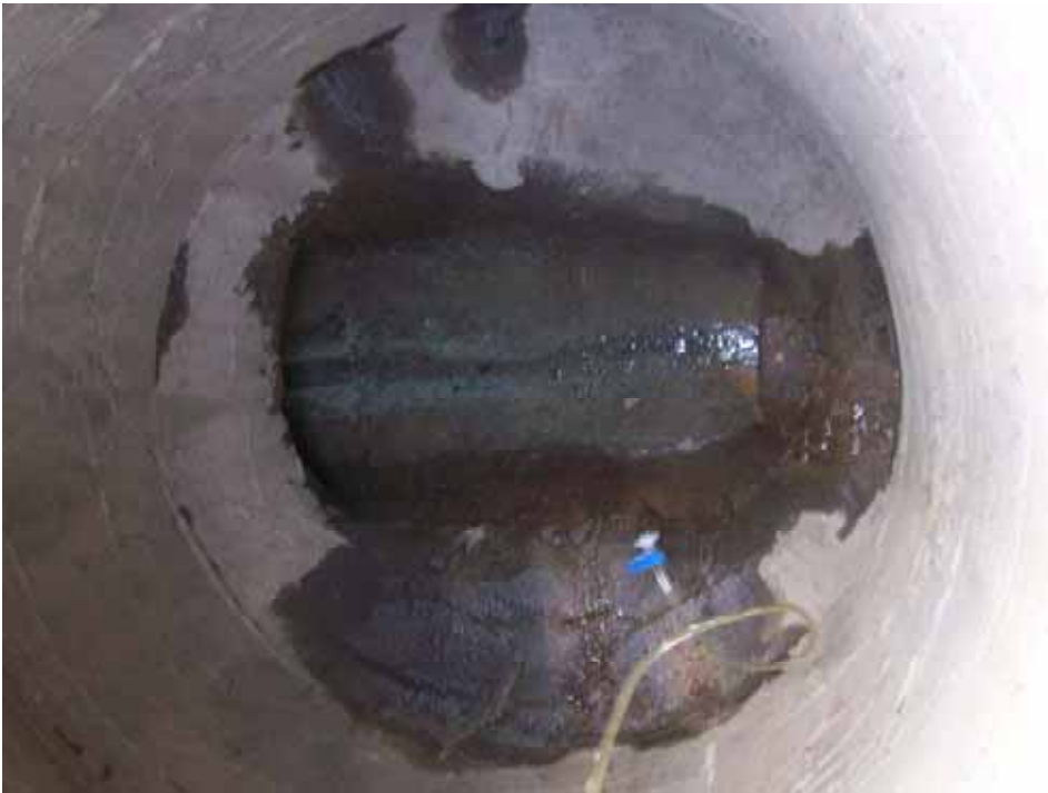
Description: Hollow Behind Coating Near FM Discharge
