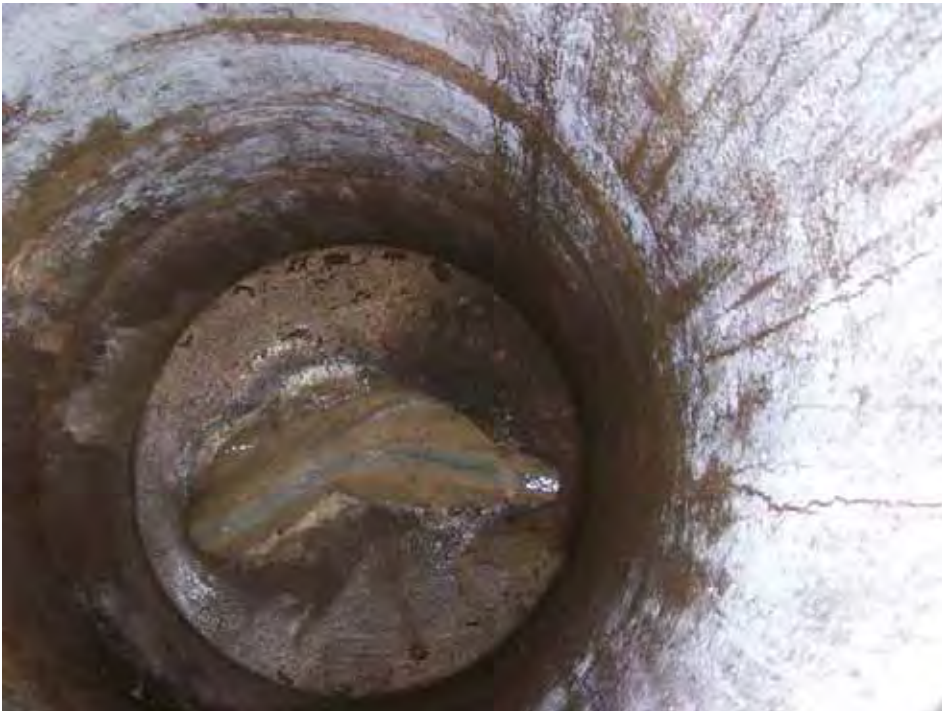
Description: White Deposits on Unlined Concrete
