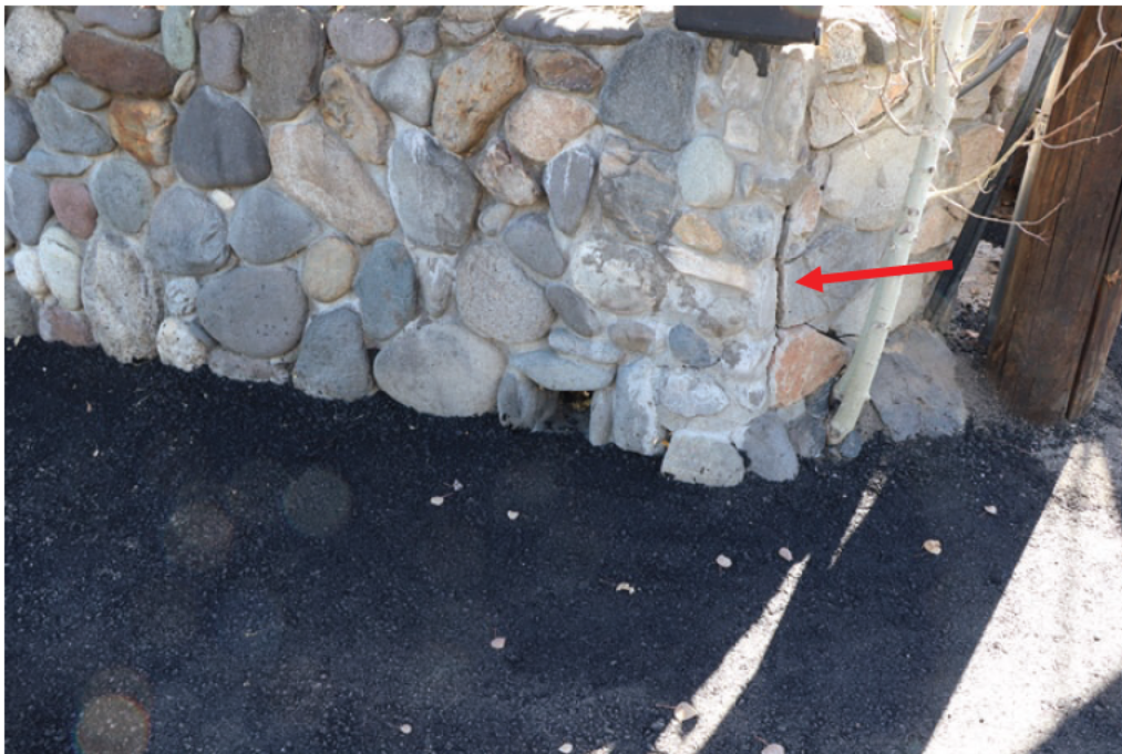
Photo 6: Closer view of the retaining wall drain outlet. Note crack in neighbor's wall (arrow).
