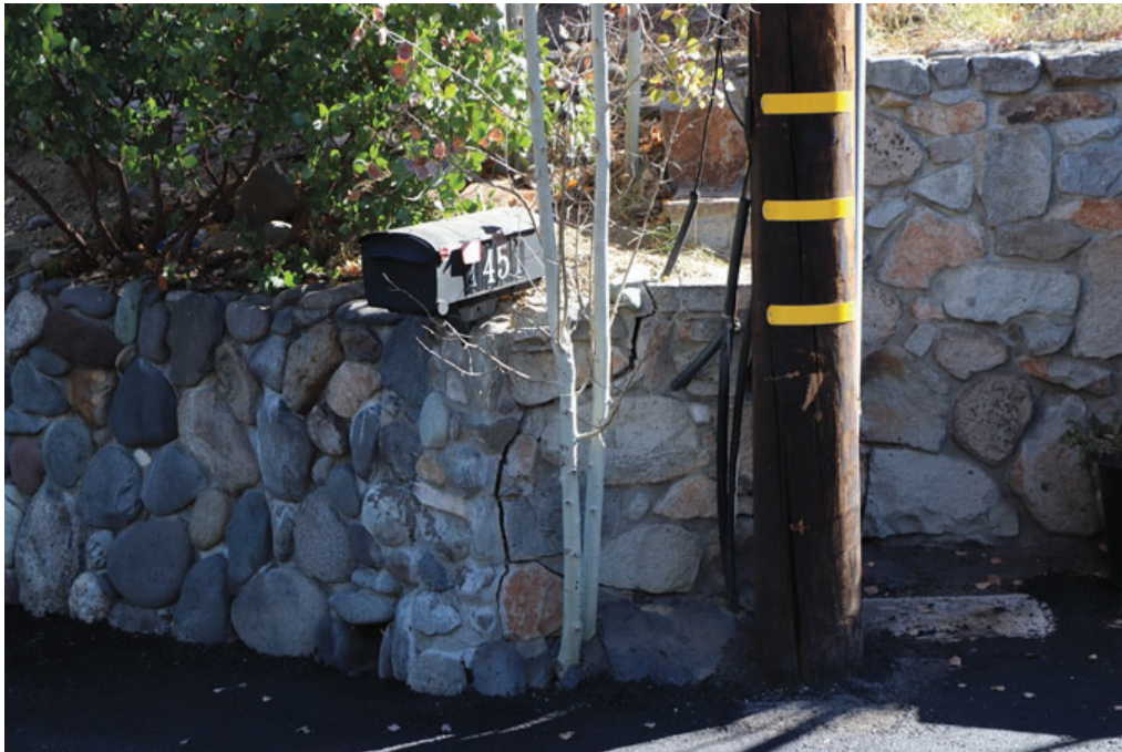
Photo 8: Crack in the neighbor's retaining wall, near where it joins the claimant's wall.
