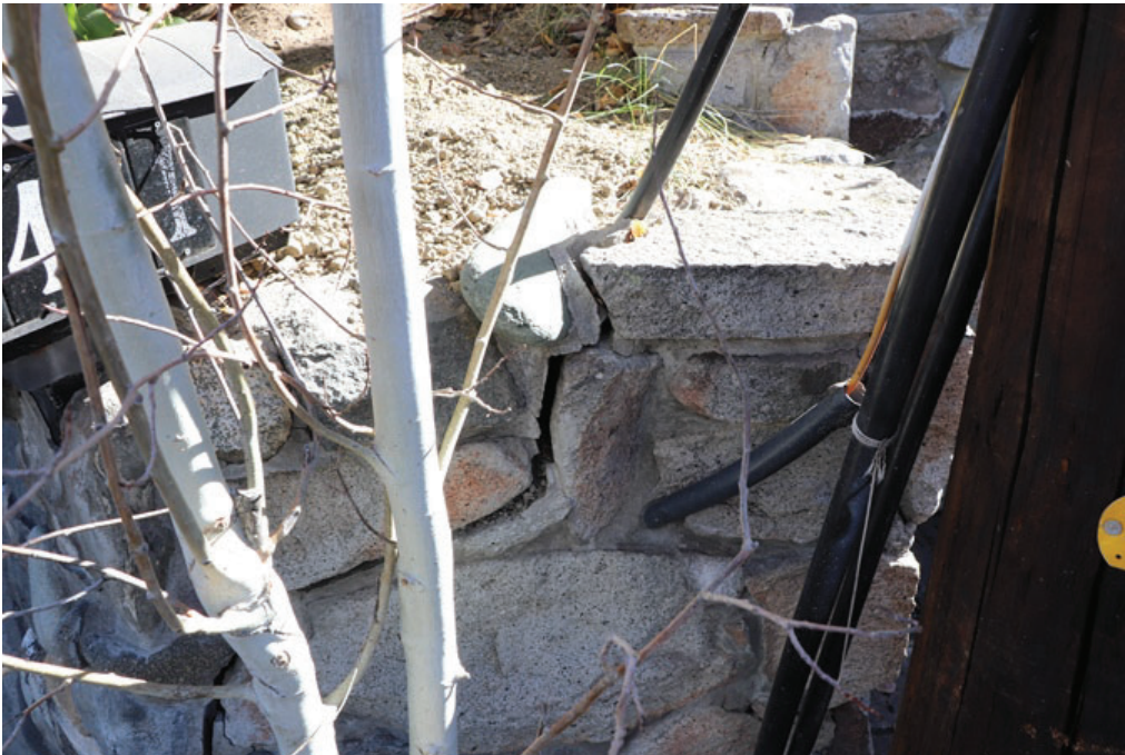
Photo 12: Panned up and right from the previous photograph. Crack in neighbor's retaining wall.
