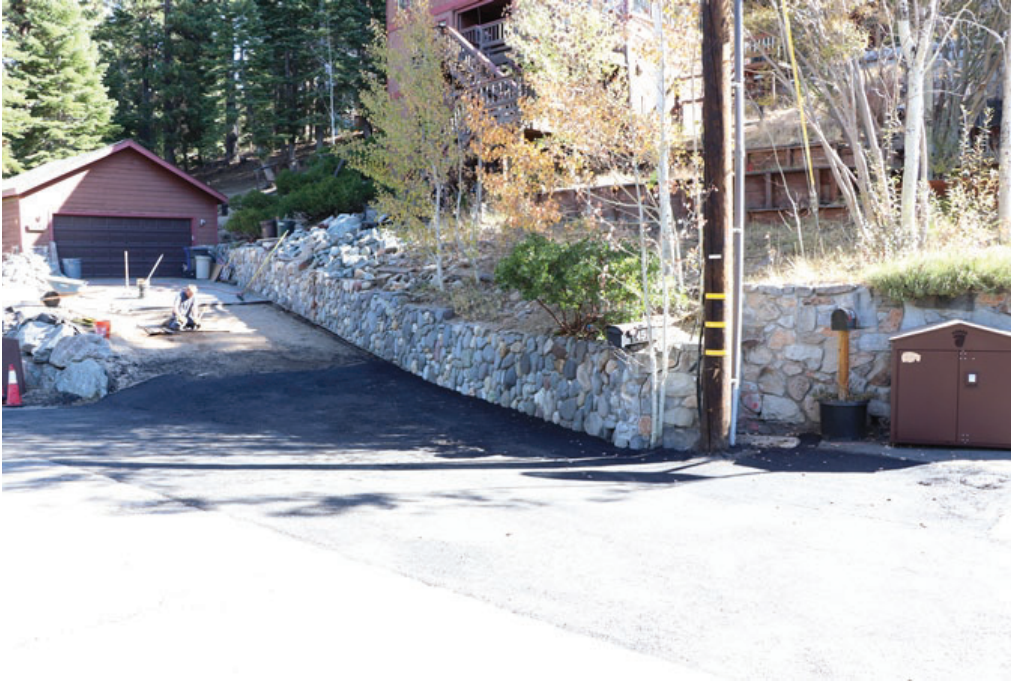
Photo 1: Overall view of the subject retaining wall to the right of the claimant's driveway.
