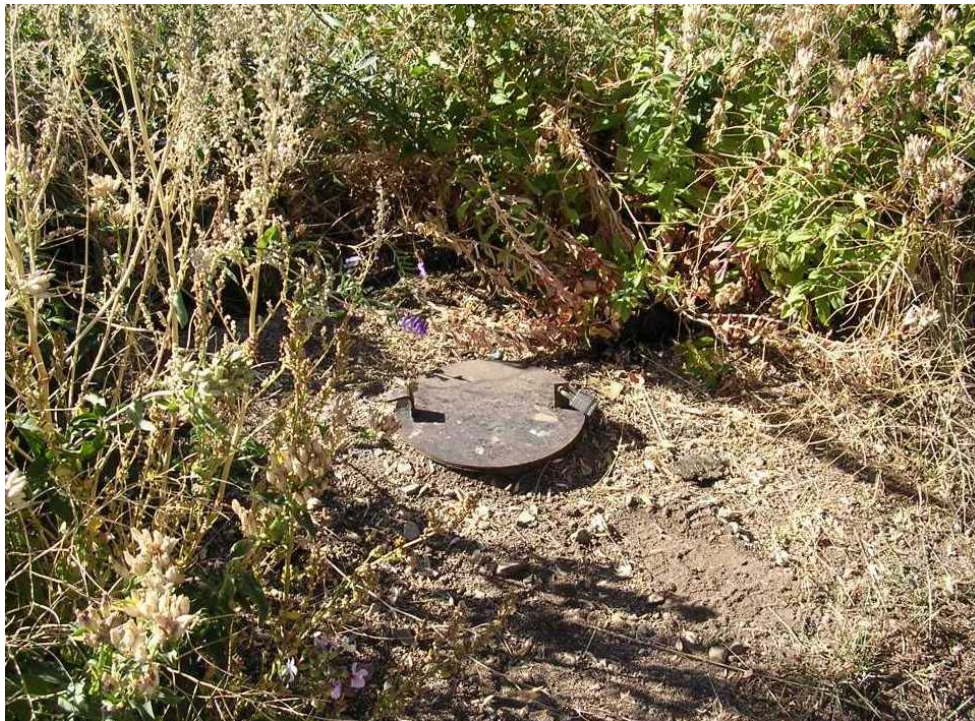
Photo of ACMW-04 with no concrete seal around wellbox
