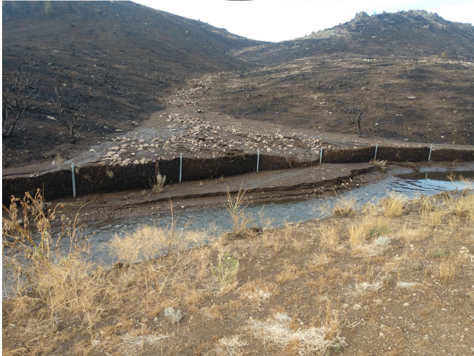
Mud slide into Diamond Ditch caused by flash floods after the Tamarack Fire.
