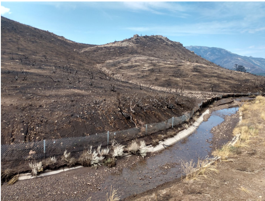
Rock, silt and burned vegetation clog 1.25 miles of Diamond Ditch after flash flooding.
