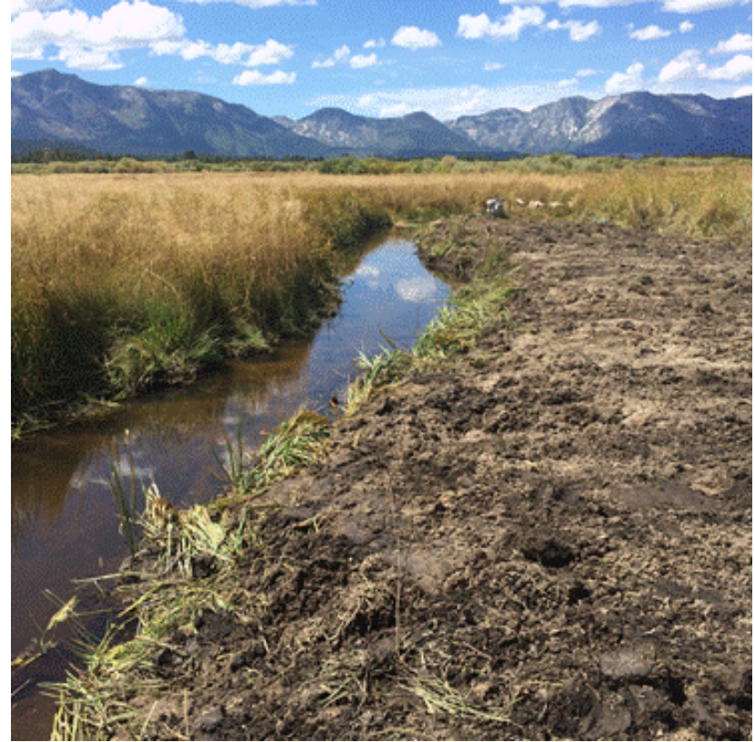
Photo 18. August 27, 2015. Hand clearing vegetation at Trout Creek to direct flows away from the pipeline ROW. Bare soils were seeded
