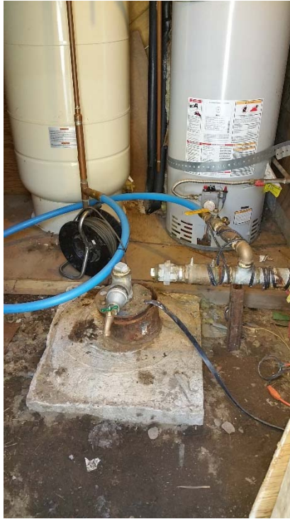
15. Transducer installed into Rockwater Well
