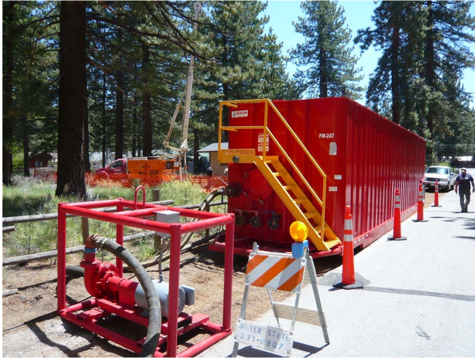
21,000 Gallon tank and Trash Pump
