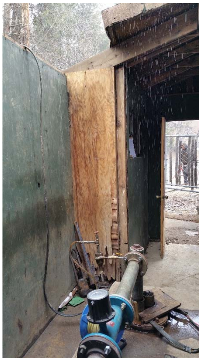
18. Flow meter at well head
