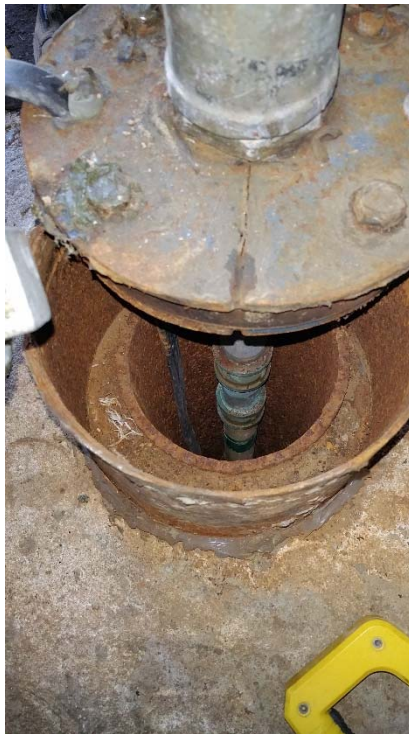
17. Rockwater Well pump column, looking down the well
