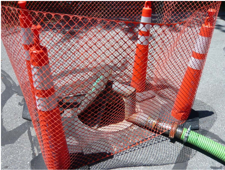
Sanitary Sewer Discharge Set-up
