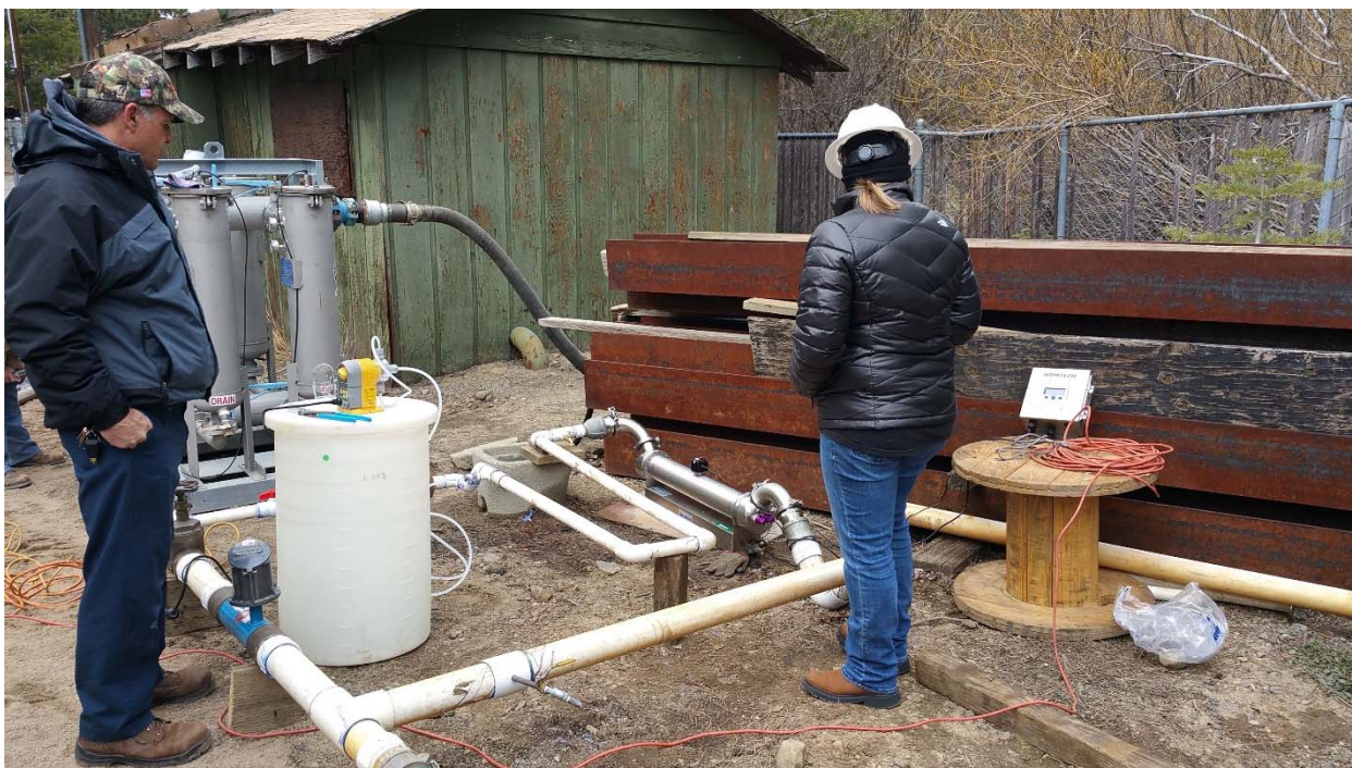
10. UV Pilot Testing with chlorine solution and chlorine pump
