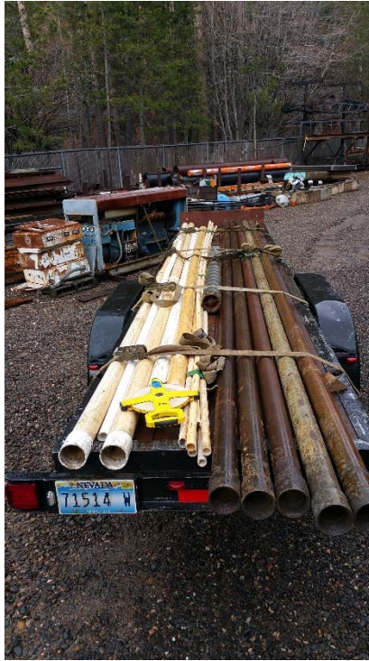
3. Column Pipe and PVC sounding tube, submersible pump and motor
