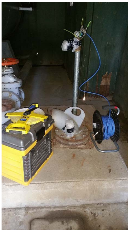
16. Pressure transducer installed into LBWC #4 Well
