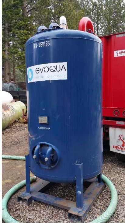
7. Evoqua PV2000 GAC vessel
