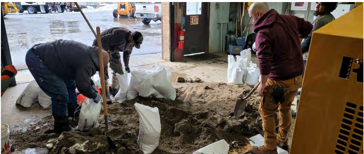
Sand bags were placed around pump stations to prevent stormwater from flowing into the sewer system.
