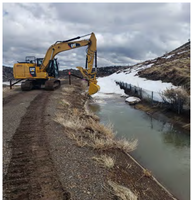
Clearing ice and debris from Diamond Ditch in advance of emergency release of recycled water from Harvey Place Reservoir.
