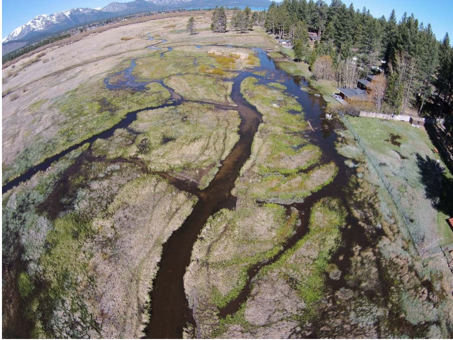
Figure 4-5. Upstream of Bellevue work area looking west, 17 Apr 2015 (pilot channels diverting flow to left overbank and right overbank plugs as disconnections in channels on right overbank)
