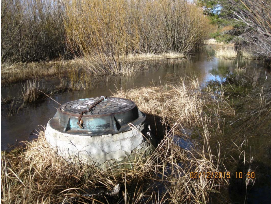
Figure 4-9. STPUD Manhole BV22, inundation due to beaver activity, 12 Feb 2015
