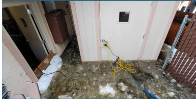
Flooding at the STPUD Bellevue Sewer Pump Station during that occurred in February 2024 and involved severe winter storms, flooding, and landslides.
