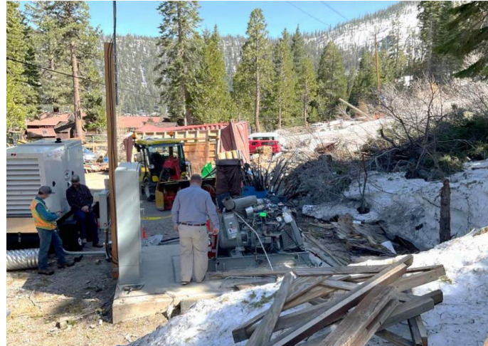
Damaged Stanford Camp Emergency Diesel Generator and Building from a 2023 Avalanche.
