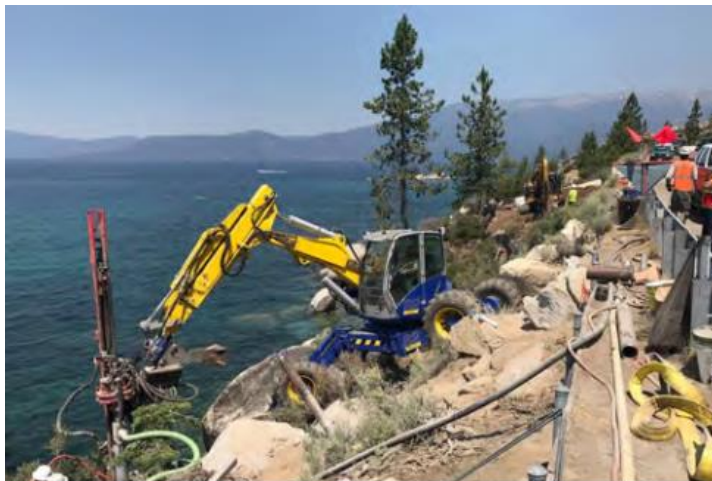
Construction along NV State Route 28. Retrofitting roads to withstand extreme weather protects people and infrastructure investments.
